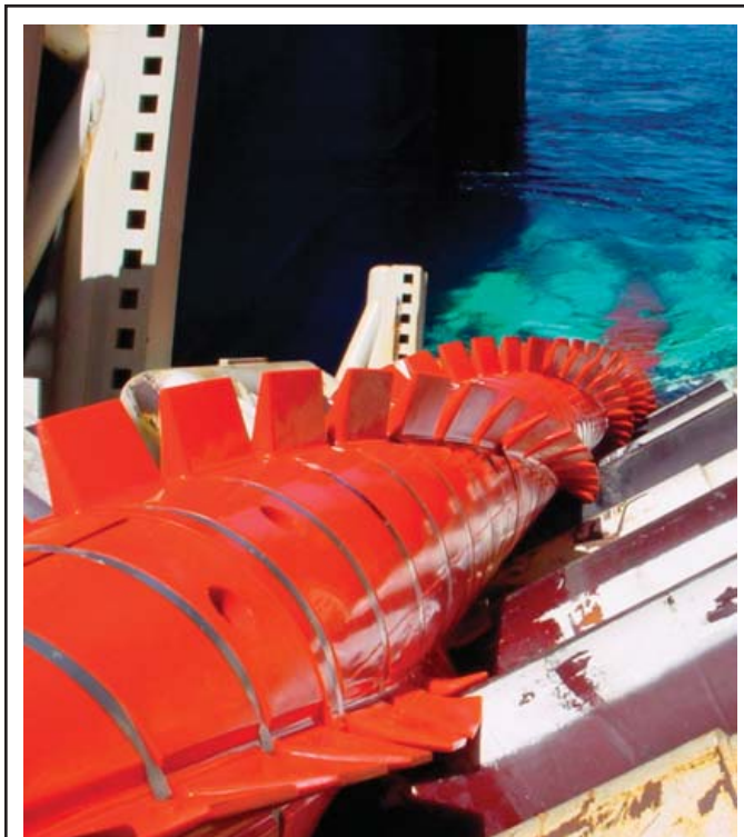
The 24-inch Independence Trail pipeline stretches 135 miles to a new shallow-water platform at West Delta 68. Allseas USA Inc.'s dynamically-positioned Solitaire —the largest pipe-lay vessel in the world—installed the pipeline after undergoing modifications required to lay the pipe and steel catenary riser in such deep water. Here, pipe leaves the Solitaire 's stinger, with a vortex induced vibration (VIV) strake attached to improve stability.
