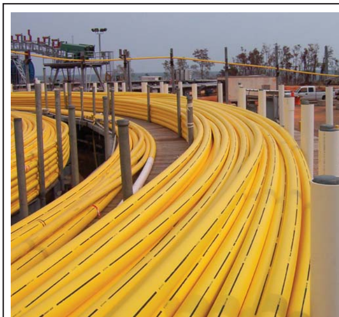
The Independence subsea system uses more than 125 miles of umbilicals—the world's largest single subsea umbilical order. It also includes 220 miles of flowlines and 155 flowline jumpers and flying leads.
