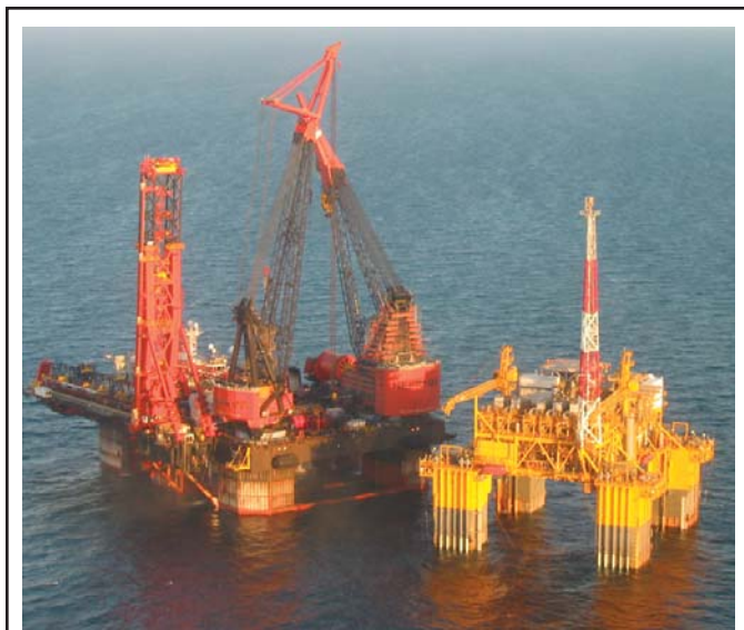
The Independence Hub is scheduled to receive first gas later this year from 15 wells in 10 fields in water depths to 9,000 feet. The semisubmersible platform is shown here on location in 8,000 feet of water at Mississippi Canyon Block 920 with Heerema's DCV Balder during installation work.
